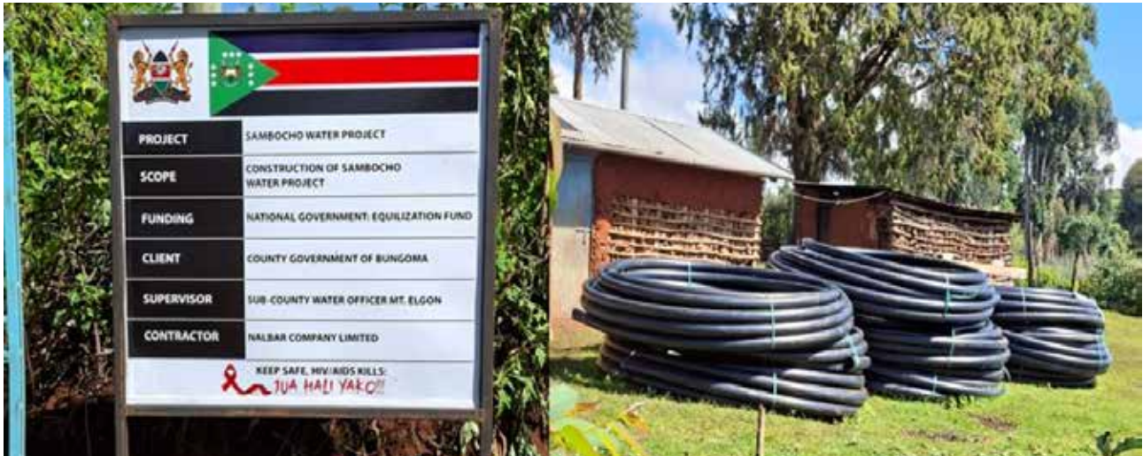
Picture 5: Publicity Signboard and water pipes for the Sambocho water project
