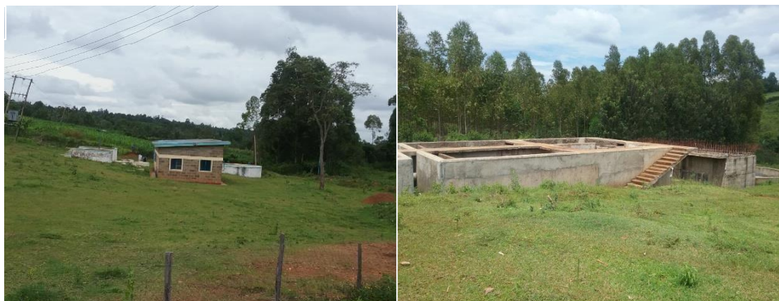
Current and Ongoing Water Treatment Plants
