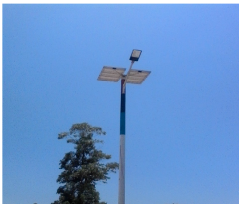
Nyang' omak solar street lights in North Sakwa
