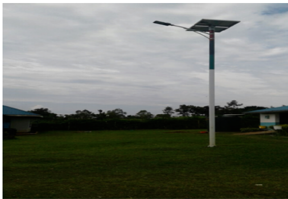
Solar lighting at Ngodhe dispensary in East kamagambo ward
