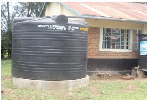
Piny owacho water tank in Central kanyamkago
